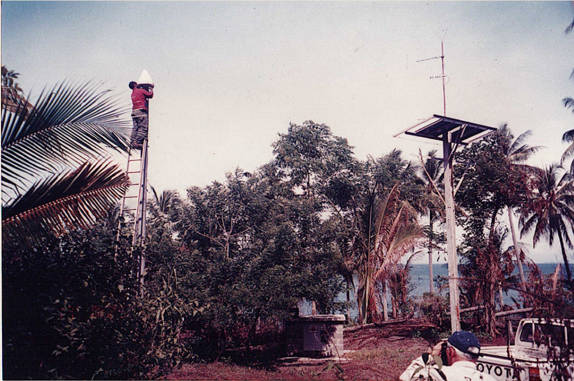
The Remote site at Vulcan Island South (VIS). A concrete bunker to house the receiver, telemetry, power etc. At left the choke ring antenna is being placed on a 6 m pole. At right a solar panel mast, with the telemetry yagi antennas. The masts are so high so as to avoid being over taken by tree growth. The opportunity was taken to co-host seismometers in the bunkers.
