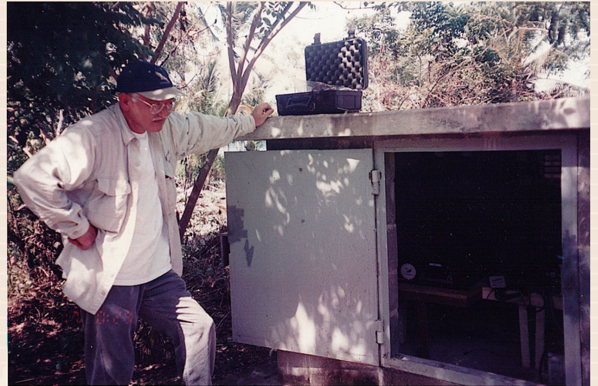
Elliot Endo inspects a bunker (1999), the Ashtech rack mount, housing the Z12 and Bel S103 radio can just be made out.
